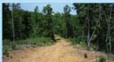
The top image is an example of a good BMP which intercepts a large ditch drain. The lower image shows the soil loss and bank damage that a poorly designed road causes. Photo by Brandon Day.
