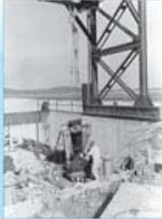
Workers install sections of the intake piping for a pump. Photo courtesy of Central Arkansas Water.
