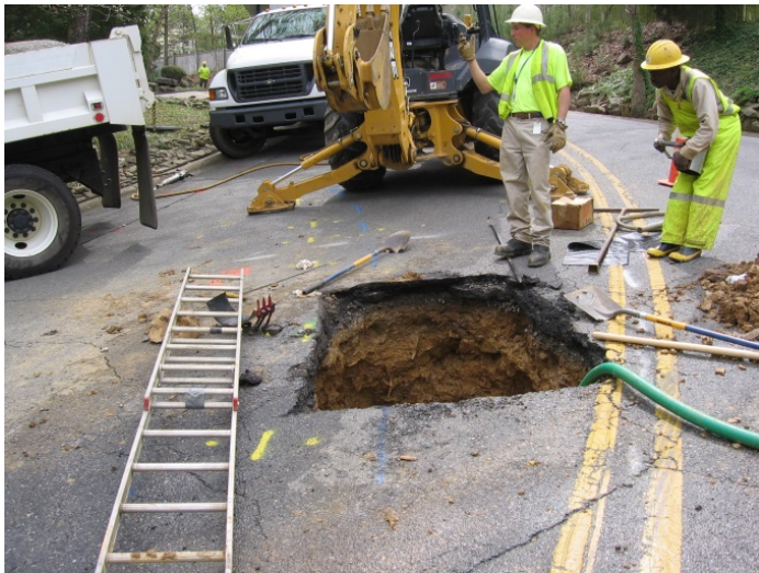
CAW crews work to repair a main with minimal disruption to customer or traffic.
