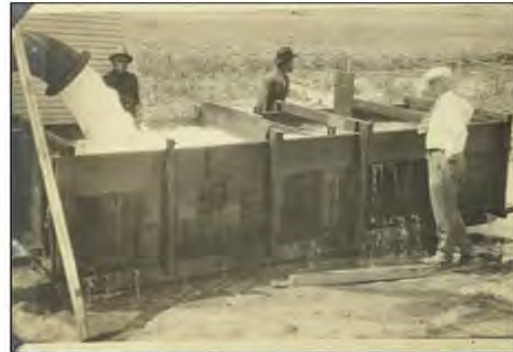
Treatment Water Well E – April 1925 – Arkansas Water Company employees try to figure out how to stop the leak.
