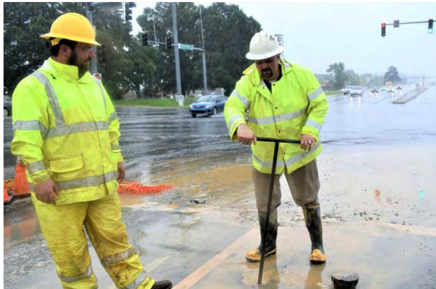
CAW Distribution personnel repair a break on University Avenue in Little Rock.
