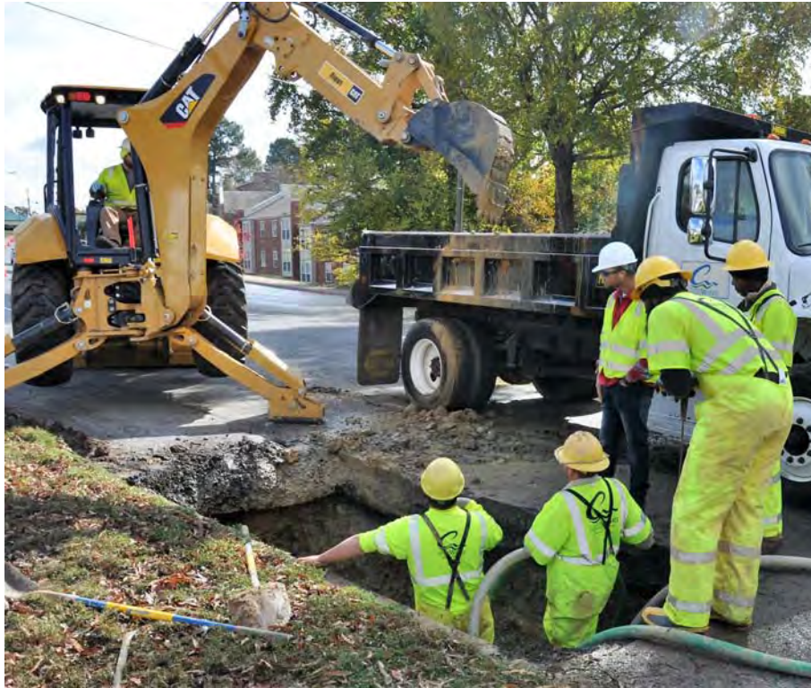
CAW Distribution crew repairing a main break on Cantrell Road in Little Rock.
